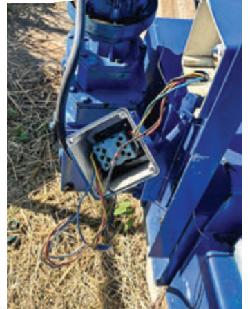
The Democratic Alliance says this photo shows damaged and exposed electrical components at the Brits sewage treatment plant, which it claims contribute to the plant's ongoing non-functionality.
